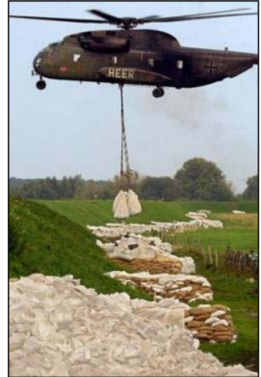
Flood prevention by dike observation
